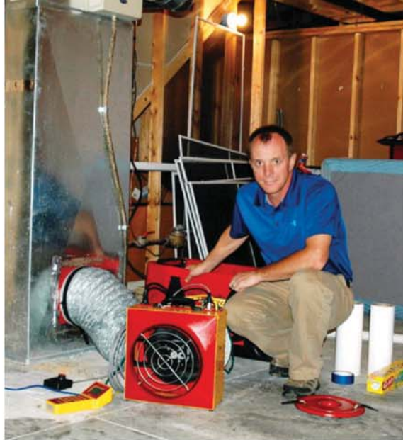
Rob Novak, chief building analyst at Home Star Iowa, checks out progress of a duct blower during a recent energy audit. Rob has conducted over 100 energy audits for his brother Randy, president of Novak Heating and Air Conditioning. Both claim energy audits help boost an average sale by 35 percent.
